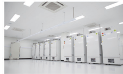
3. Preservation room (Deep Freezer)
